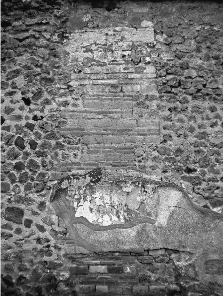
Plate 3.2 Repairs in brick to the north enclosure wall of the Temple of Apollo
