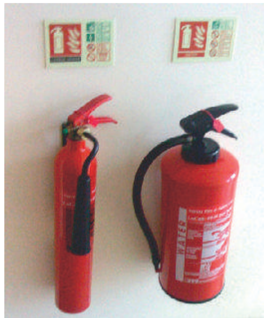
Figure 1.44 CO 2 and water extinguishers and information posters
