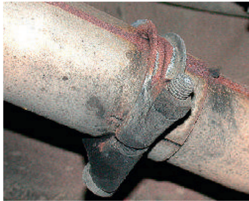
Figure 1.71 Corrosion on an exhaust joint
