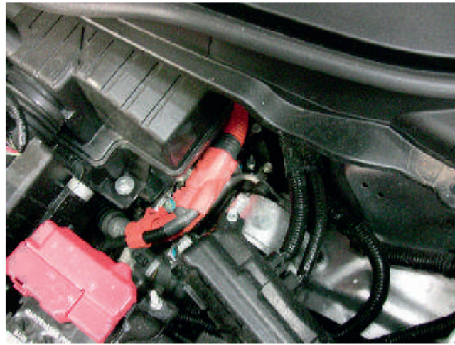
Figure 2.345 High-voltage cables are always orange
