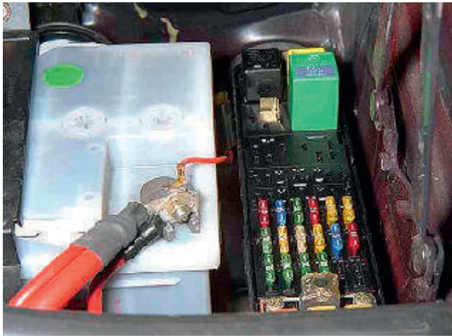
Figure 3.51 Correct polarity is important: red cables are used for the positive connection
